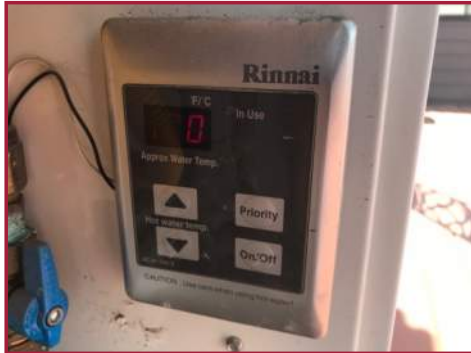
THERMOSTAT TO WATER HEATER IN ROOFTOP WATER HEATER CABINET
