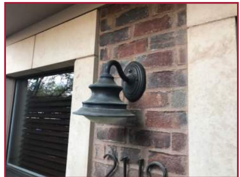
INOPERATIVE LIGHT FIXTURE AT FRONT PORCH/ENTRY
