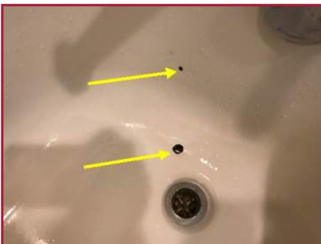
BATHTUB HAS SURFACE DAMAGE IN DOWNSTAIRS BEDROOM BATHROOM
