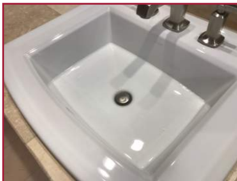
SINK DRAINS SLOWLY AT SOUTH VANITY IN MASTER BATHROOM
