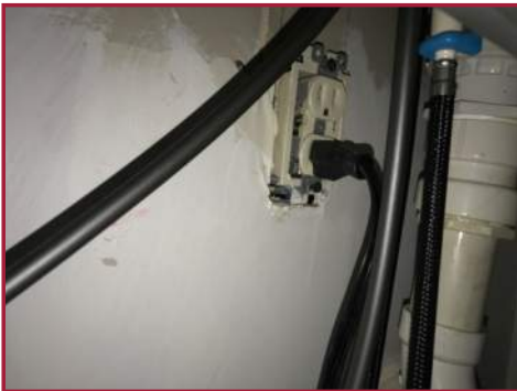
MISSING RECEPTACLE COVER UNDER KITCHEN SINK
