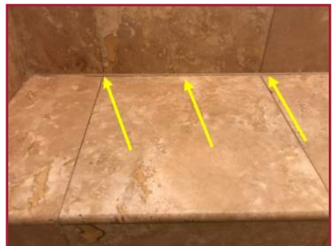
CRACKED/DETERIORATED SHOWER GROUT IN MASTER BATHROOM
