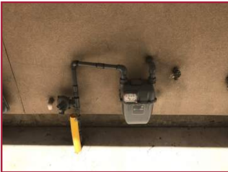
GAS METER ON SOUTH SIDE OF STRUCTURE
