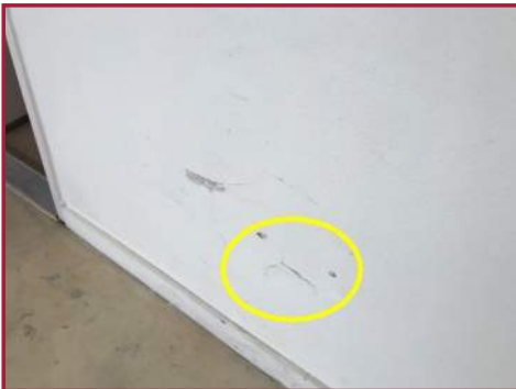
IMPACT DAMAGE IN GARAGE
