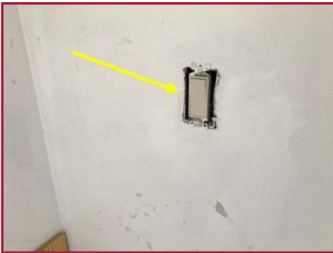
MISSING SWITCH PLATE COVER IN ROOFTOP STORAGE CLOSET
