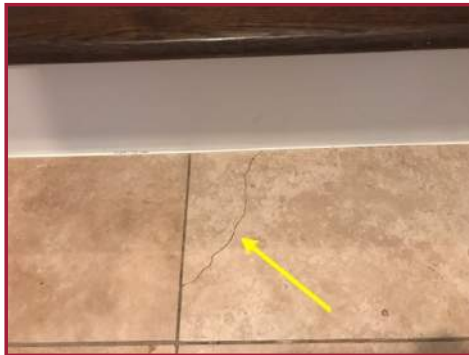
CRACKED/DAMAGED FLOOR TILE AT BASE OF FIRST FLOOR STAIRWAY
