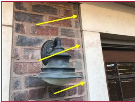
MINOR CRACKS IN MORTAR AROUND CAST STONE ENTRY
