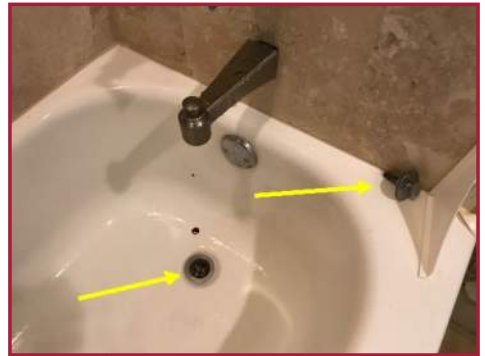
STOPPER IS DAMAGED TO DOWNSTAIRS BEDROOM BATHTUB
