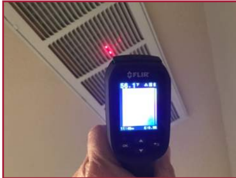
AMBIENT TEMPERATURE AT DOWNSTAIRS HVAC RETURN AIR VENT DURING TEST
