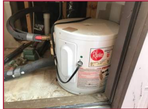
ANCILLARY WATER HEATER
