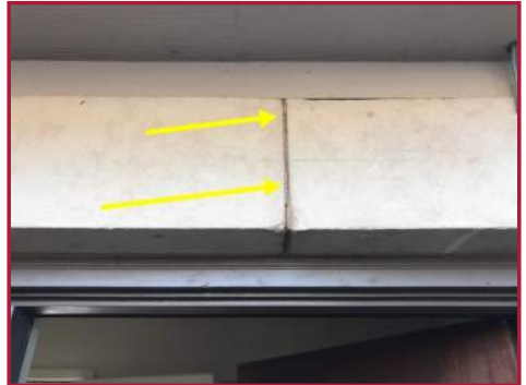
CRACK IN CAST STONE GROUT OVER FRONT ENTRY
