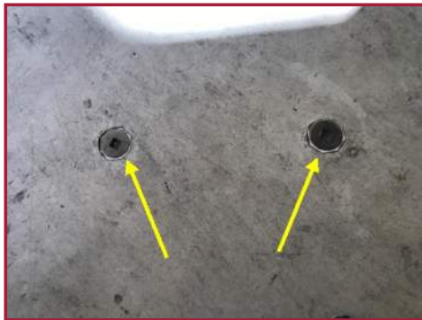
SEWER CLEANOUTS IN GARAGE
