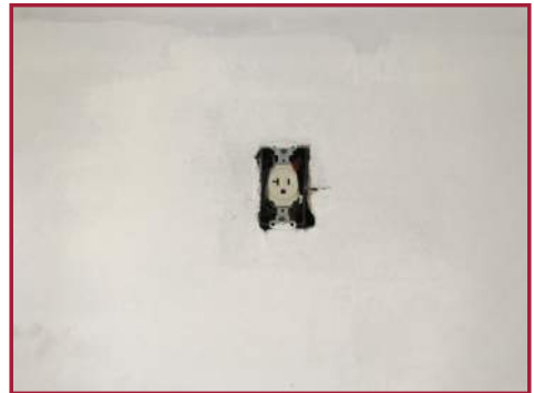
MISSING RECEPTACLE COVER IN ROOFTOP STORAGE CLOSET
