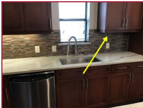
INOPERATIVE LIGHT FIXTURE RIGHT OF KITCHEN SINK
