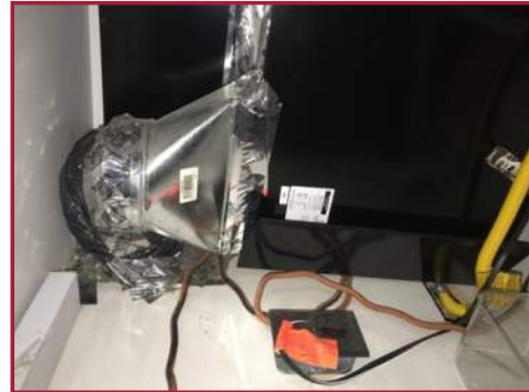
DUCTWORK ON DOWNDRAFT VENT HOOD
