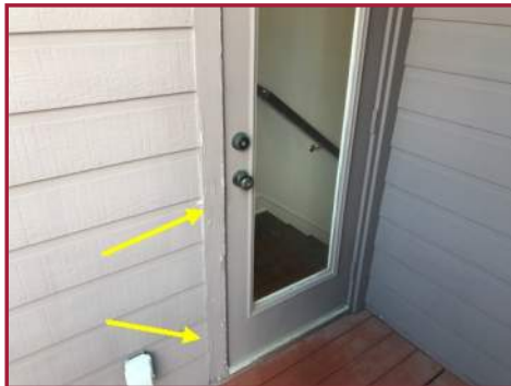
PAINT NEEDED AROUND DOOR JAMB TO ROOFTOP DECK
