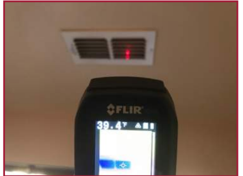
AMBIENT TEMPERATURE AT DOWNSTAIRS HVAC SUPPLY VENT DURING TEST
