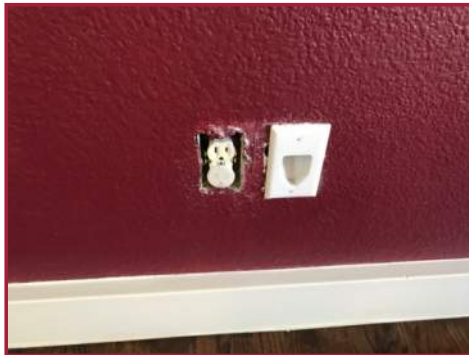
MISSING RECEPTACLE COVER IN LIVING ROOM
