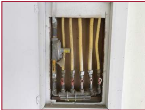
CSST GAS PIPING MANIFOLD
