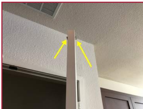
DAMAGED SPRING LATCH TO PANTRY DOOR
