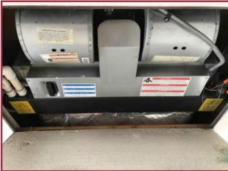
DOWNSTAIRS CENTRAL HEATING SYSTEM UNIT
