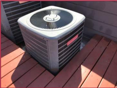
DOWNSTAIRS CENTRAL COOLING UNIT
