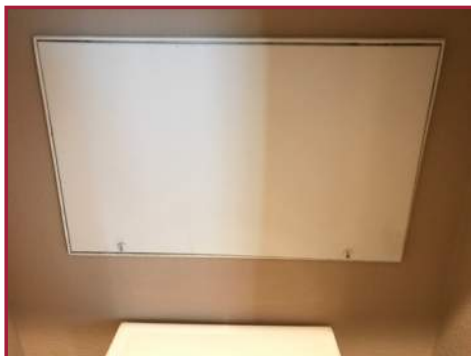
ACCESS TO DUCT DAMPER VALVES OVER MASTER TOILET
