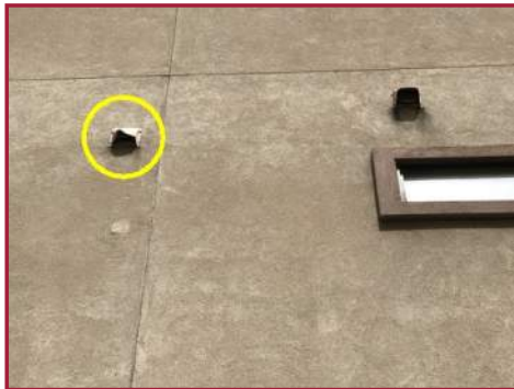
DAMAGED EXHAUST VENT ON SOUTH SIDE OF STRUCTURE
