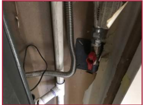
NO SEDIMENT TRAP ON UPSTAIRS UNIT
