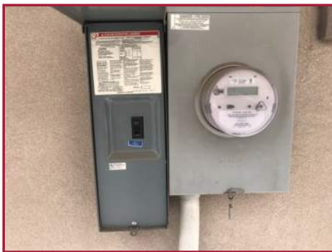
MAIN SERVICE DISCONNECT ON SOUTH EXTERIOR WALL
