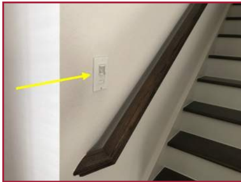
MOTION DETECTOR ON SECOND LEVEL STAIRWAY NOT PERFORMING CORRECTLY
