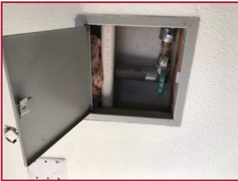
MAIN WATER VALVE IN GARAGE
