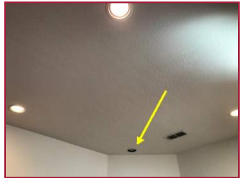
INOPERATIVE LIGHT FIXTURE IN STUDY
