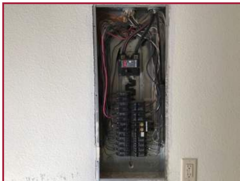
MAIN PANEL WITH COVER REMOVED FOR INSPECTION
