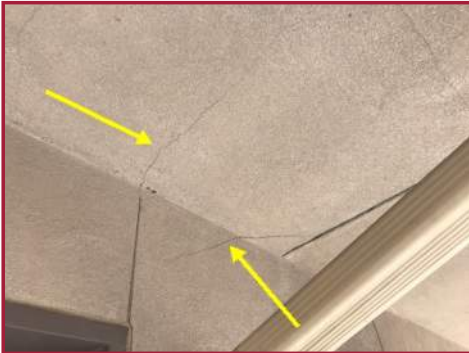
CRACKS IN EIFS STUCCO OVER EAST SIDE OF GARAGE DOOR
