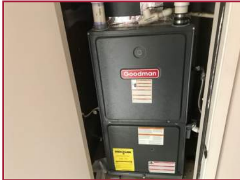
UPSTAIRS CENTRAL HEATING SYSTEM UNIT
