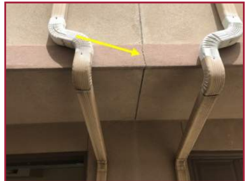
CRACK IN EIFS STUCCO BAND OVER EAST SIDE OF GARAGE DOOR
