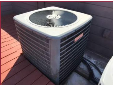
UPSTAIRS CENTRAL COOLING UNIT
