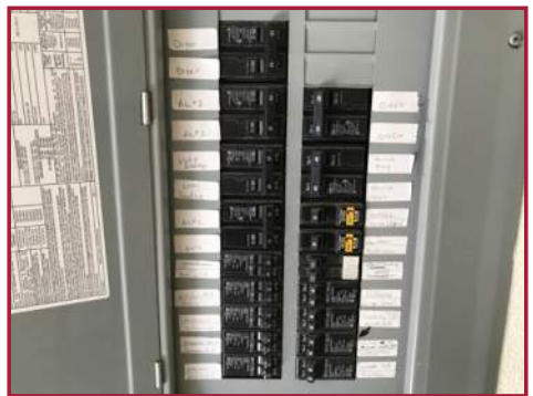
BREAKERS ARE PROPERLY LABELED
