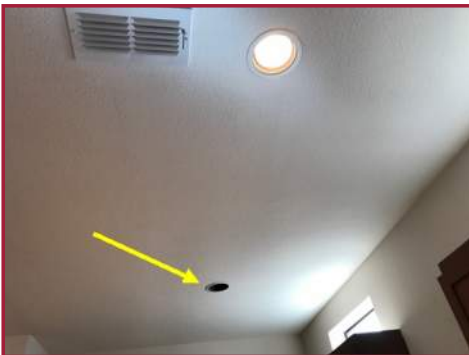
INOPERATIVE LIGHT FIXTURE IN KITCHEN
