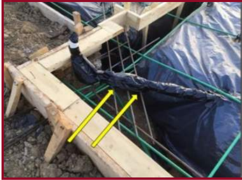
PLUMBING IN CONTACT WITH REBAR
