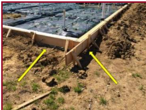
FILL NEEDED AROUND FORMS
