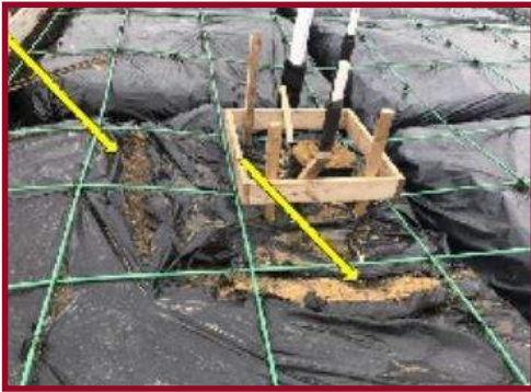
TEARS IN MOISTURE BARRIER
