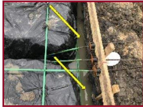
WATER IN BEAM
