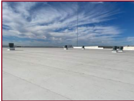
ROOF EXHAUSE FANS
