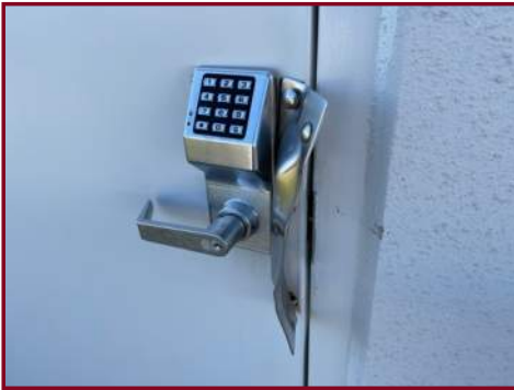
DOOR TO FIRE RISER ROOM HAS BEEN VANDALIZED
