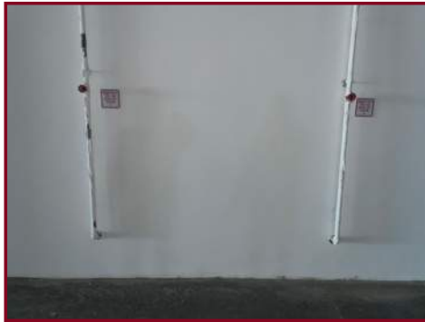
FIRE SPRINKLER INSPECTOR'S TEST STATION #2 & 3
