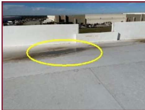
STANDING WATER ON WEST SIDE
