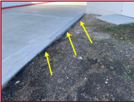
FILL DIRT REQUIRED AGAINST CURB AT NORTHEAST CORNER
