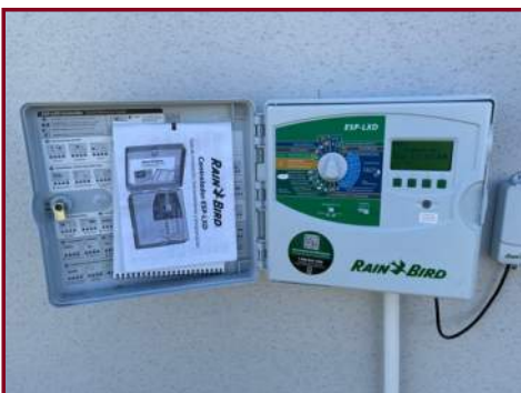
IRRIGATION SYSTEM CONTROL BOX
