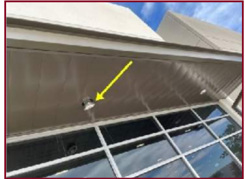
LOOSE RECESSED SPOTLIGHT IN MAIN ENTRANCE AWNING
