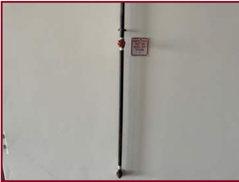
FIRE SPRINKLER INSPECTOR'S TEST STATION #1
