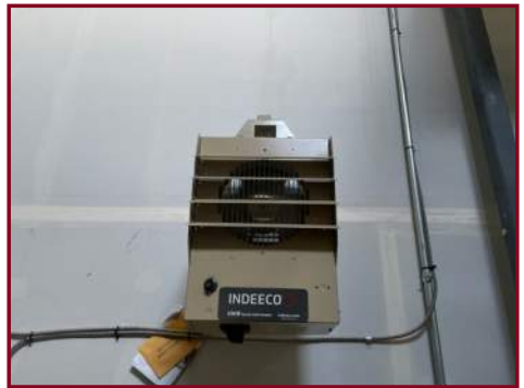
FIRE PUMP ROOM HEATER
