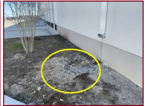
EROSION UNDER ROOF DOWNSPOUT NEAR NORTHEAST CORNER
