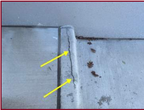
CRACKED/DAMAGED CURB RIGHT OF FIRE RISER ROOM
