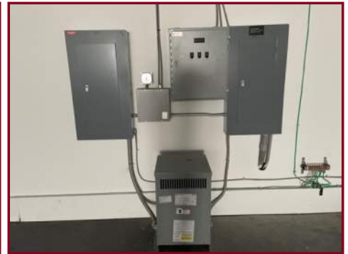
BREAKER PANELS AND STEP DOWN TRANSFORMER
