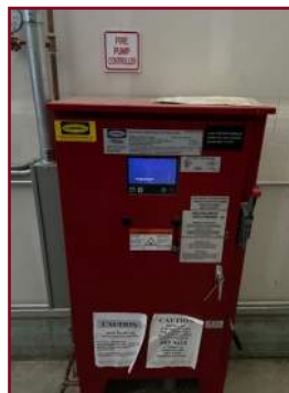
FIRE PUMP CONTROLLER
