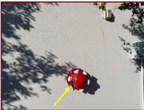
FIREMAN'S EXTERIOR HOOK-UP ON EAST WALL IS LEAKING WATER
