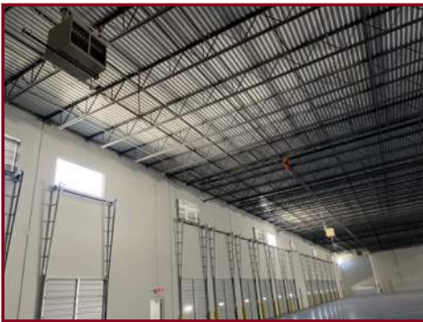
SUSPENDED WAREHOUSE HEATERS
