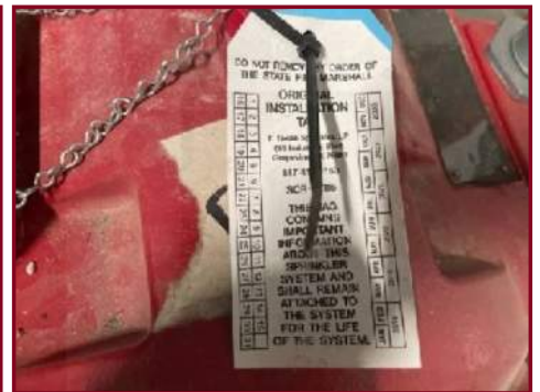
FIRE SPRINKLER TAGS SHOWED NO INSPECTION
