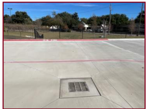
STORM DRAIN IN EAST DRIVE
