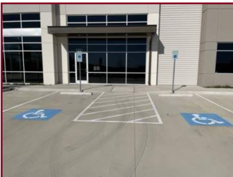
HANDICAP PARKING AT MAIN ENTRANCE
