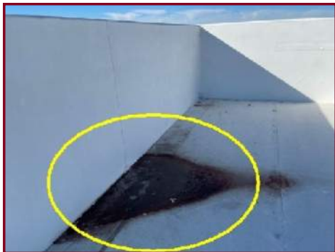
STANDING WATER AT SOUTHWEST CORNER
