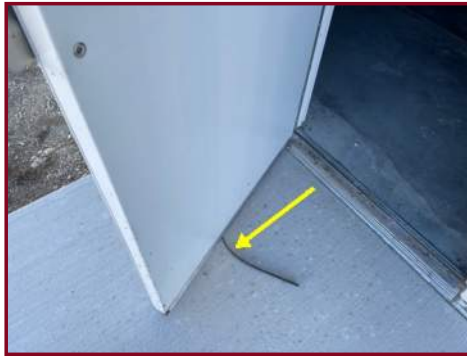
DAMAGED WEATHERSTRIPPING AT NORTHEAST EXIT DOOR
