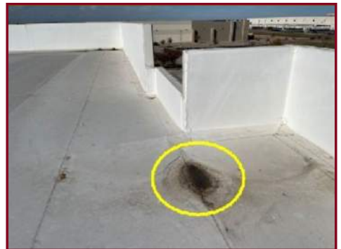
STANDING WATER ON NORTH SIDE
