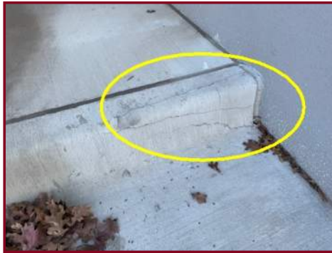
CRACKED/DAMAGED CURB RIGHT OF FIRE RISER ROOM
