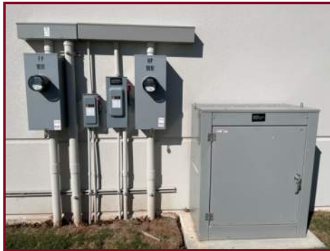
SERVICE ENTRANCE PANELS
