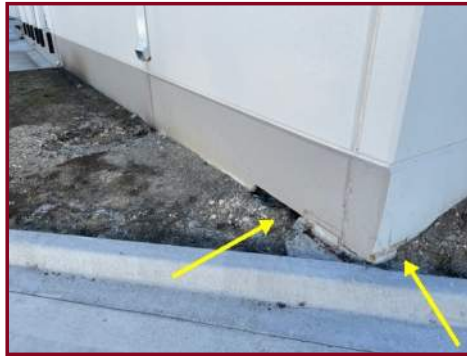
EROSION AT NORTHEAST CORNER FOUNDATION
