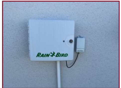
IRRIGATION SYSTEM CONTROL BOX
