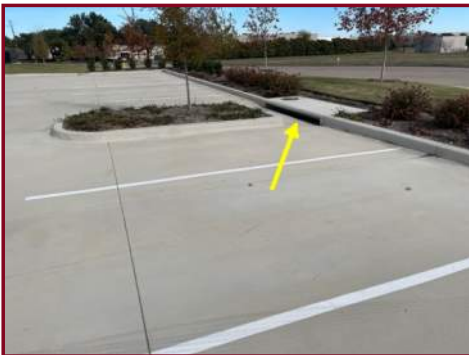
STORM WATER DRAIN IN FRONT PARKING LOT
