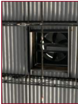
TYPICAL ROOF EXHAUST FAN
