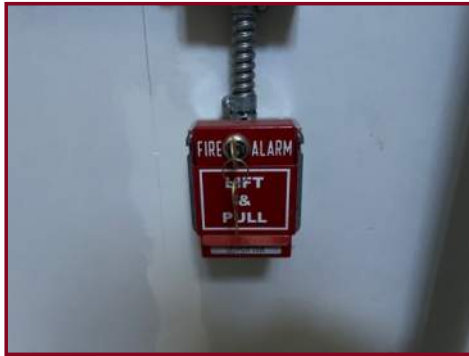
TYPICAL PULL STATION
