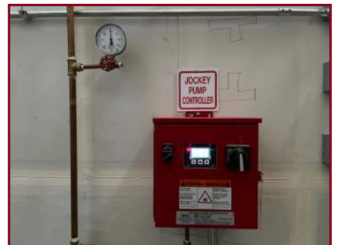
JOCKEY PUMP CONTROLLER
