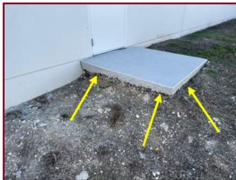
EROSION UNDER NORTHEAST EXIT DOOR STOOP
