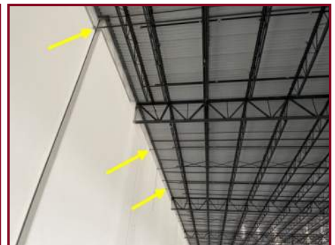
HORIZONTAL BRIDGING IS PROPERLY TIED TO EXTERIOR WALLS
