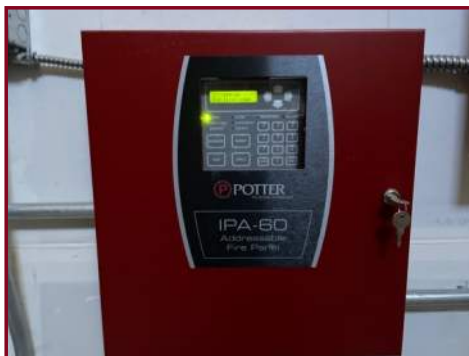
SPRINKLER ALARM CONTROLS
