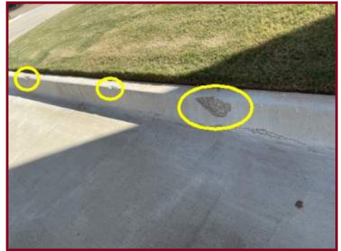
DAMAGED CURB AT SOUTH END OF TRUCK BAY DRIVE
