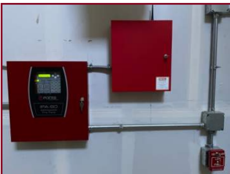
SPRINKLER ALARM CONTROLS
