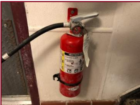
TYPICAL FIRE EXTINGUISHER
