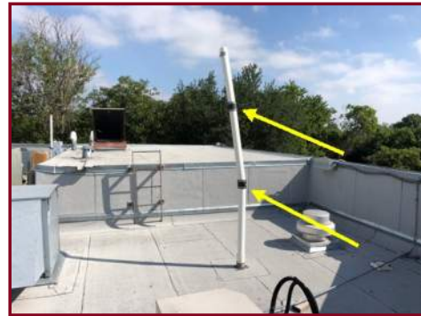
PLUMBING VENT NEEDS PROPER PVC COUPLINGS
