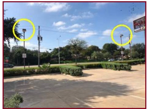
POLE MOUNTED FIXTURES
