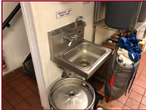
HAND WASH SINK
