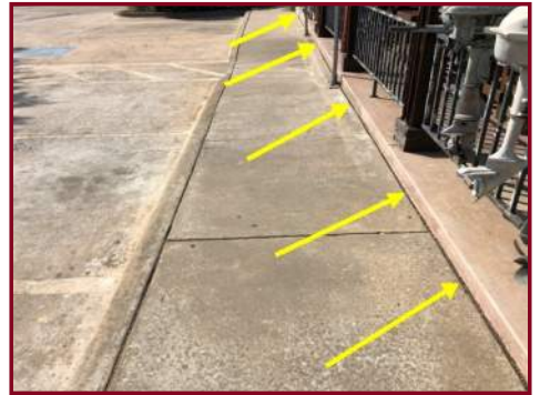
JOINT BETWEEN PATIO AND SIDEWALK SHOULD BE SEALED
