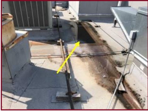
STANDING WATER ON ROOF
