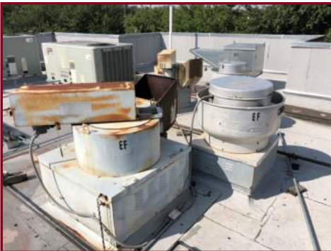
KITCHEN EQUIPMENT VENT FANS
