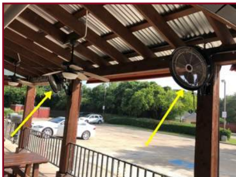
MIST FANS UNDER COVERED DINING AREA
