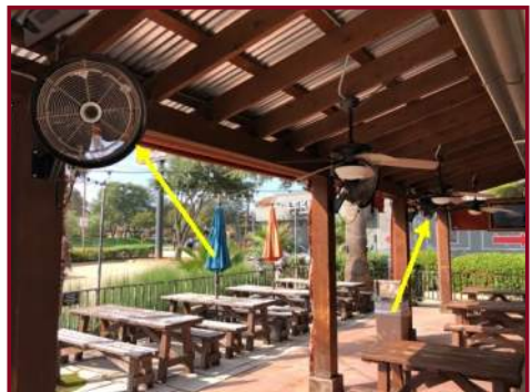
MIST FANS UNDER COVERED DINING AREA
