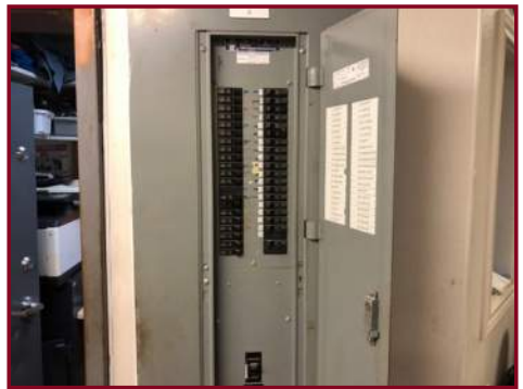
BREAKER PANEL "A"
