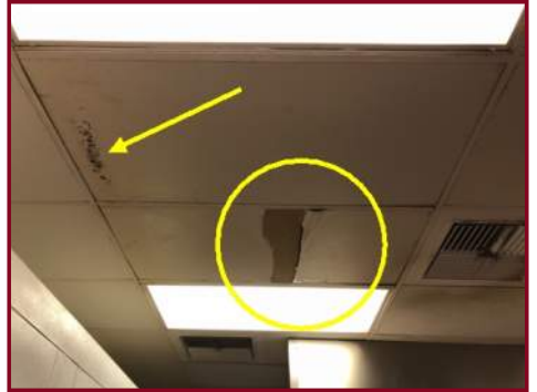
MOISTURE DAMAGED CEILING TILES IN KITCHEN
