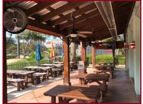
SOFFIT MOUNTED FIXTURES
