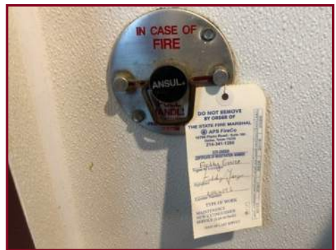
KITCHEN VENT HOOD FIRE SUPPRESSION PULL STATION
