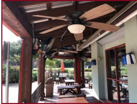
SOFFIT MOUNTED FIXTURES
