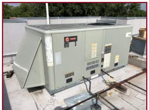
ROOFTOP PACKAGE UNIT #3
