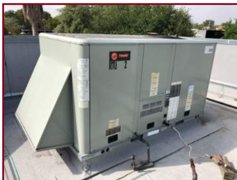
ROOFTOP PACKAGE UNIT #2
