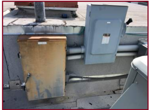
ROOFTOP EQUIPMENT DISCONNECTS
