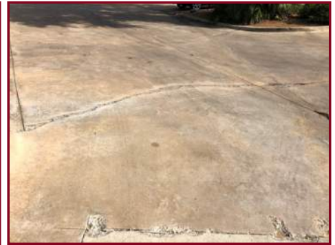
MINOR CRACKS IN PAVEMENT
