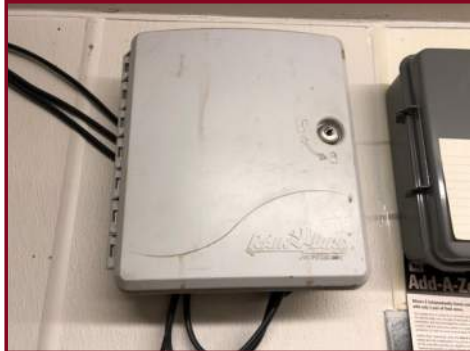
IRRIGATION SYSTEM CONTROL BOX
