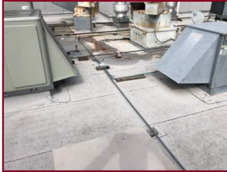
STANDING WATER ON ROOF
