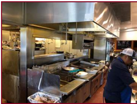
KITCHEN EXHAUST VENT
