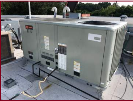
ROOFTOP PACKAGE UNIT #4
