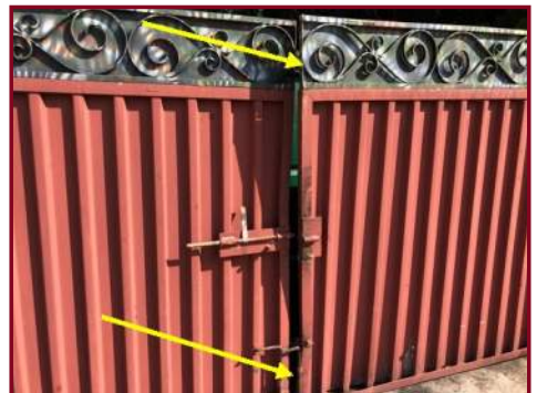
GATES ARE SPRUNG AND OUT OF ALIGNMENT
