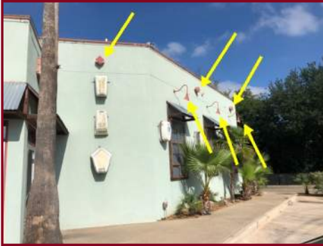
WALL MOUNTED FIXTURES
