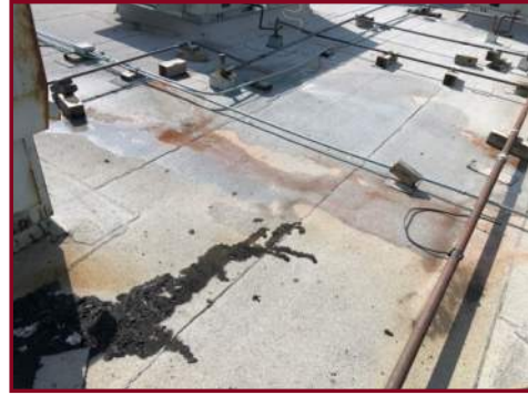
STANDING WATER ON ROOF
