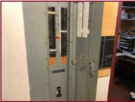
BREAKER PANEL "B"
