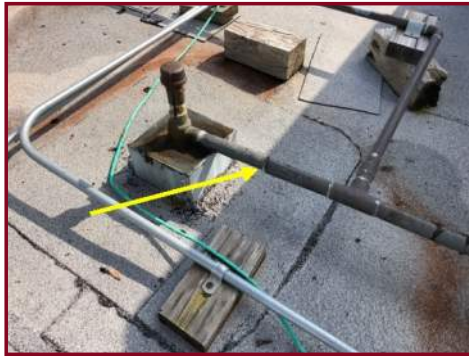
CONDENSATE DRAIN HAS BEEN CUT
