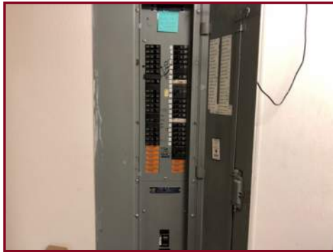
BREAKER PANEL "C"
