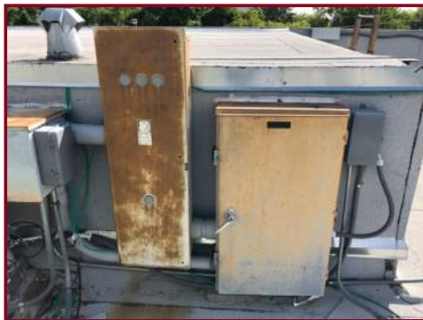
ROOFTOP EQUIPMENT DISCONNECTS
