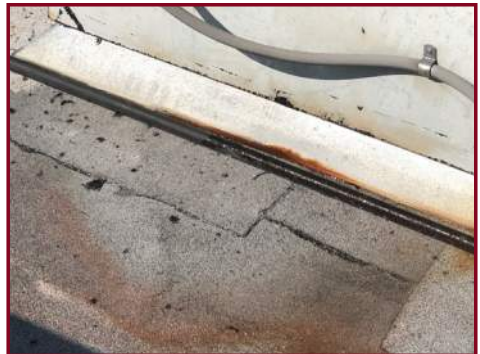
HVAC CONDENSATE LINES LEAKING ON ROOF
