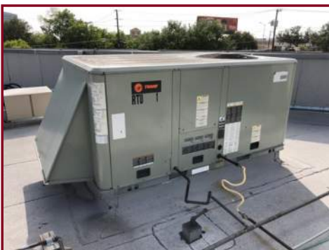
ROOFTOP PACKAGE UNIT #1
