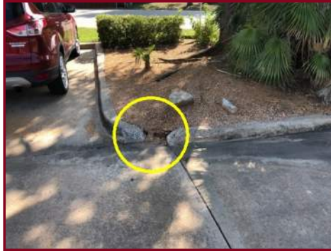
DAMAGED CURB ADJACENT TO ENTRANCE DRIVE
