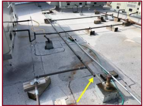
CONDENSATE DRAIN HAS BEEN CUT
