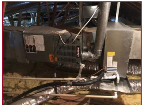
CENTRAL HEATING SYSTEM UNIT #3
