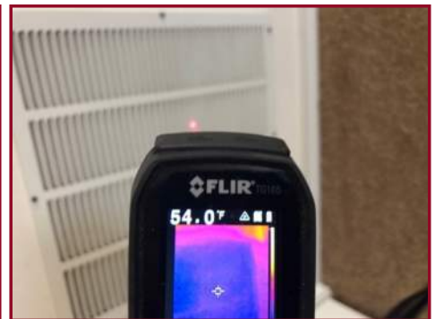
AMBIENT TEMPERATURE AT UPSTAIRS HVAC RETURN AIR VENT DURING TEST
