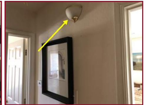
INOPERATIVE LIGHT FIXTURE IN BEDROOM HALLWAY
