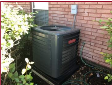
CENTRAL COOLING SYSTEM UNIT #3
