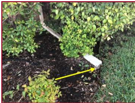
DAMAGED DOWNSPOUT EXTENSION
