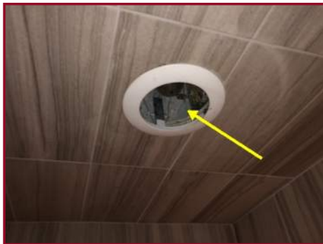
LENSE TO THE CAN LIGHT IS MISSING IN MASTER BATHROOM SHOWER
