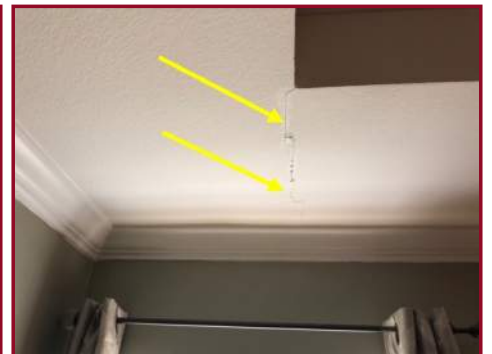
CEILING STRESS CRACKS IN MASTER BEDROOM
