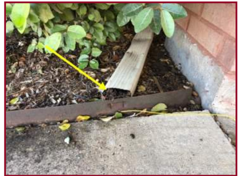
DOWNSPOUT IS CLOGGED ON NORTH SIDE
