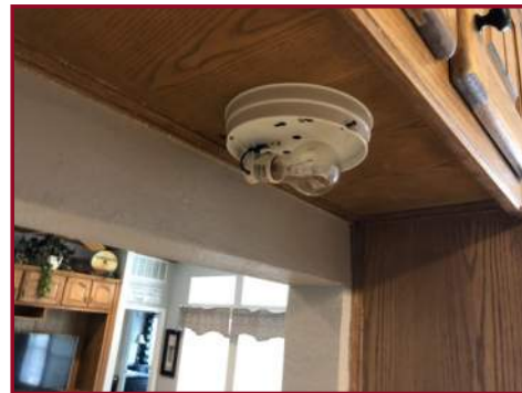
MISSING COVER TO LIGHT FIXTURE OVER KITCHEN SINK
