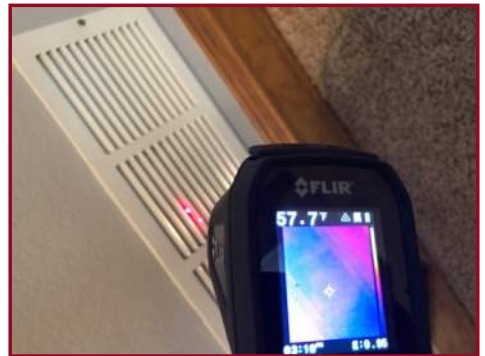
AMBIENT TEMPERATURE AT SOUTH BEDROOMS HVAC RETURN AIR VENT DURING TEST
