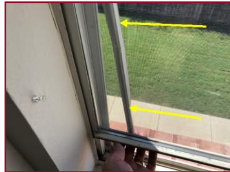
GLAZING BEAD LOOSE ON WEST WINDOW IN GAME ROOM
