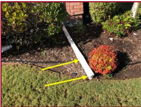
GUTTER EXTENSION DAMAGED
