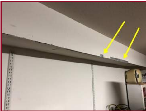
CORNER BEAD PLASTER FLAKING IN GARAGE
