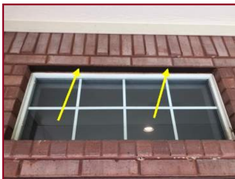
STEEL LINTELS NEED PAINT
