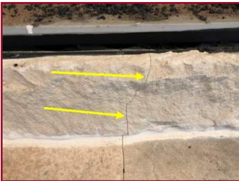
CRACK ON FACE OF FIREPLACE BELOW FIREBOX
