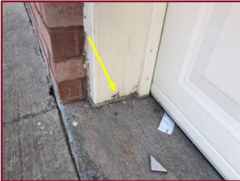
GARAGE DOOR TRIM DAMAGE
