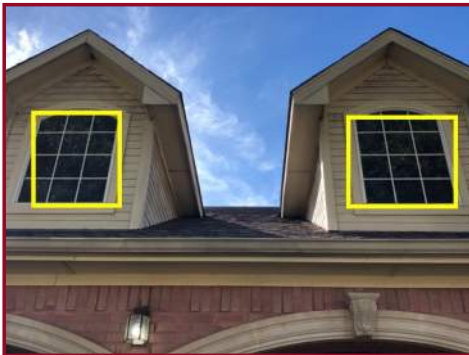
WINDOWS HAVE LOST SEAL
