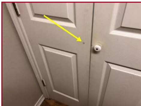
HARDWARE MISSING ON DOORS TO MASTER BEDROOM HALLWAY
