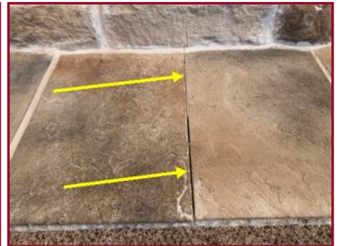
CRACKED/DETERIORATED GROUT ON HEARTH
