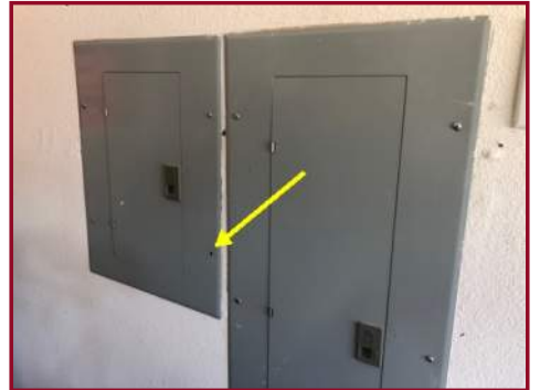
COVER PLATE MISSING SCREWS
