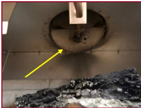
DAMPER CLAMP NEEDED
