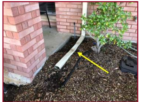
DAMAGED DOWNSPOUT EXTENSION
