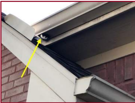
GUTTER NEEDS CLEANING
