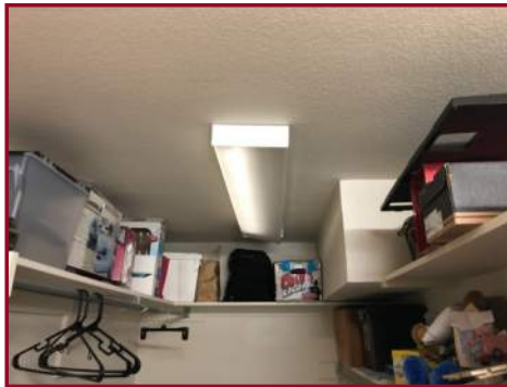
INOPERATIVE LIGHT FIXTURE IN MASTER CLOSET
