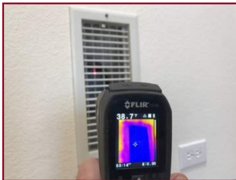
AMBIENT TEMPERATURE AT UPSTAIRS HVAC SUPPLY VENT DURING TEST
