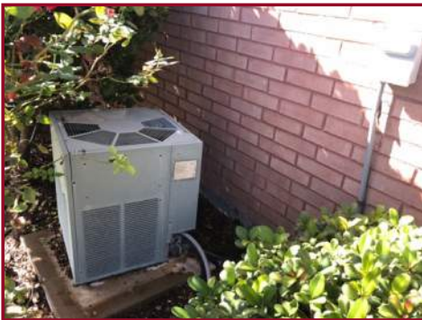
CENTRAL COOLING SYSTEM UNIT #1
