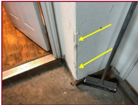
CORNER BEAD MISSING IN GARAGE
