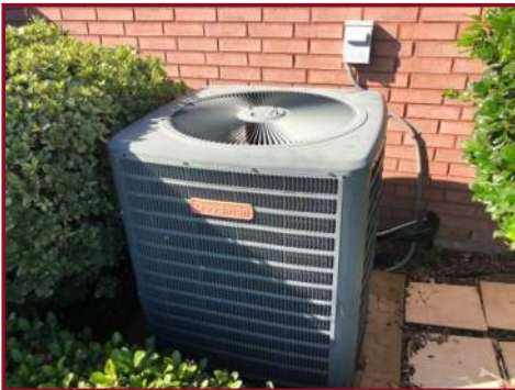
CENTRAL COOLING SYSTEM UNIT #2
