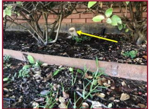
SEWER CLEANOUT ON NORTH SIDE OVERFLOWING
