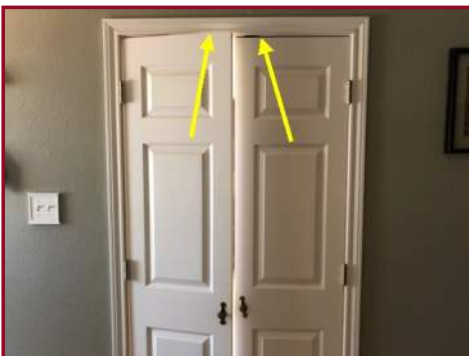
SPRING LATCH NOT FUNCTIONING PROPERLY ON MASTER BATHROOM DOORS
