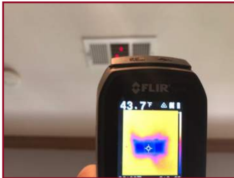
AMBIENT TEMPERATURE AT MAIN HOUSE HVAC SUPPLY VENT DURING TEST
