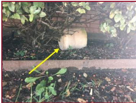
EXTRA CONCRETE CYLINDER APPARANTLY LEFT OVER FROM PREVIOUS FOUNDATION REPAIR
