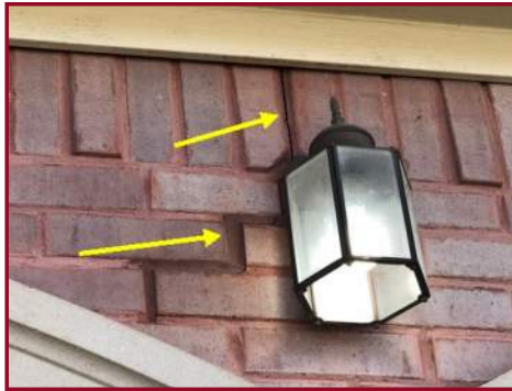
MORTAR CRACKS ON EAST SIDE
