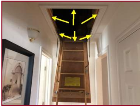
WEATHERSTRIPPING NEEDED AROUND ATTIC LADDER OPENING
