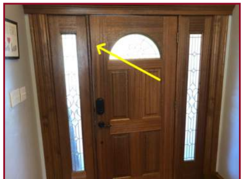
DOOR IS RUBBING THE JAMB TO THE FRONT ENTRY
