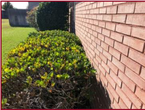
HEAVY FOLIAGE SHOULD BE TRIMMED BACK AWAY FROM WALL
