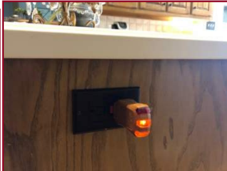
GFCI NOT WORKING PROPERLY ON CENTER ISLAND IN KITCHEN
