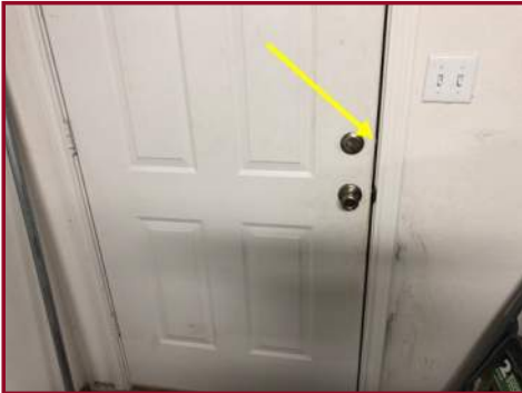
DEADBOLT NOT LATCHING PROPERLY ON GARAGE REAR ENTRY
