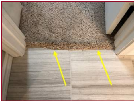
CARPETING NEEDS TO BE STRETCHED AND TUCKED AT MASTER CLOSET DOOR
