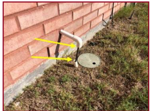
DAMAGED CONTROL WIRE CONDUIT
