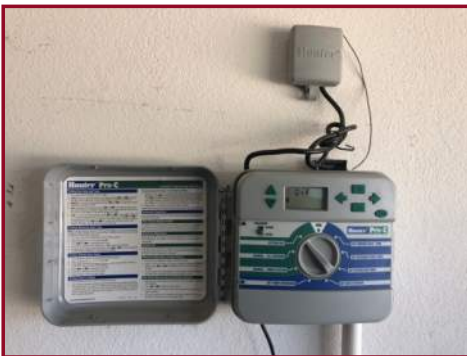
SPRINKLER SYSTEM CONTROL BOX
