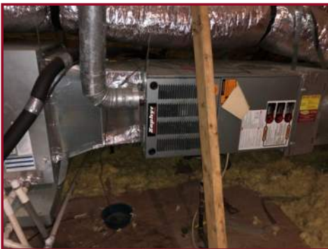
CENTRAL HEATING SYSTEM UNIT #1
