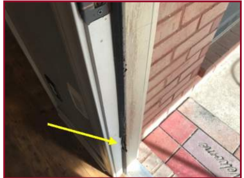
WEATHERSTRIPPING DAMAGED/MISSING ON REAR ENTRY DOOR
