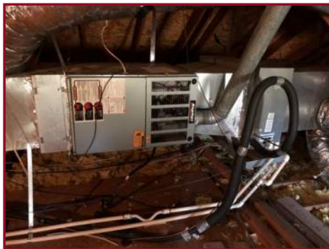
CENTRAL HEATING SYSTEM UNIT #2
