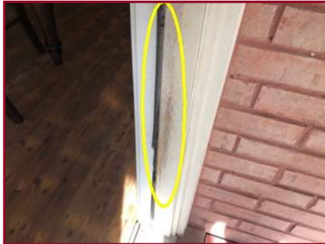
DOOR FRAME DAMAGE ON REAR ENTRY DOOR
