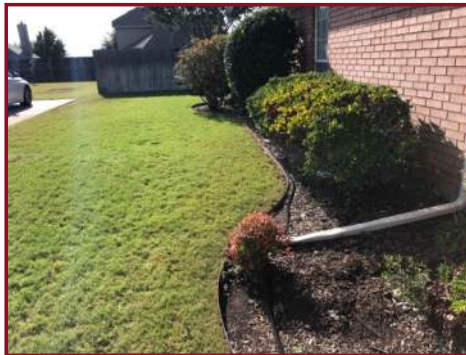
SOIL LINE IS MARGINALLY HIGH ON SOUTH SIDE OF HOUSE
