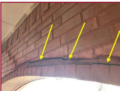
MORTAR CRACKS AT ARCH OVER FRONT PORCH
