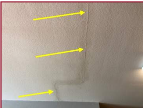
CEILING STRESS CRACKS IN KITCHEN
