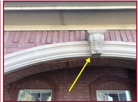
ARCH ON FRONT PORCH IS SAGGING
