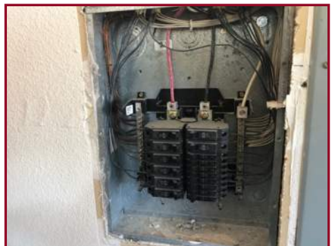
SUB PANEL WITH COVER REMOVED FOR INSPECTION PURPOSES
