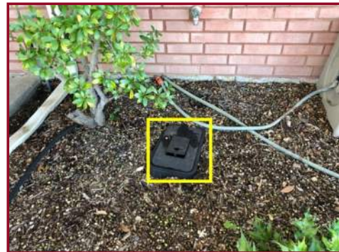
MAIN WATER VALVE IN FRONT FLOWERBED
