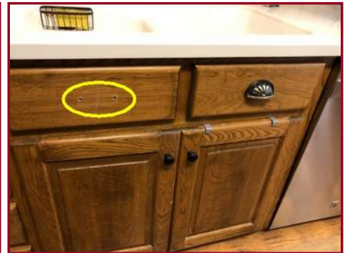
MISSING CABINET HARDWARE IN KITCHEN
