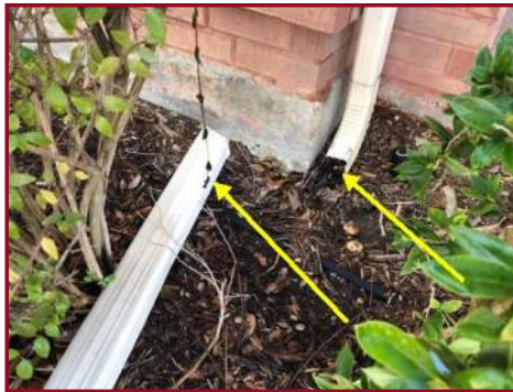
DOWNSPOUT SEPARATED AND CLOGGED WITH LEAVES ON EAST SIDE
