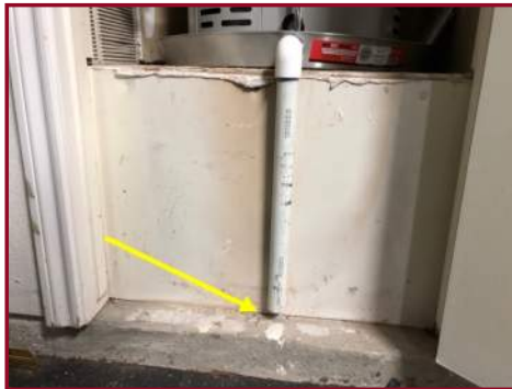
PAN DRAIN LINE TERMINATES IN GARAGE
