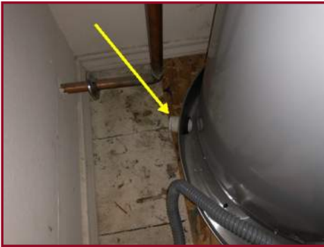
NO DRAIN LINE ON DRAIN PAN
