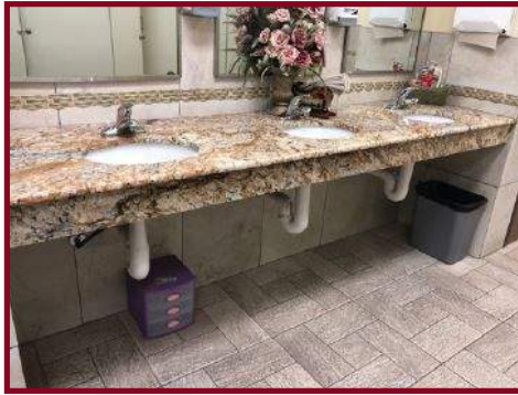
PUBLIC ADA SINKS
