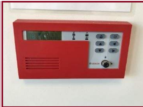
ALARM KEY PAD
