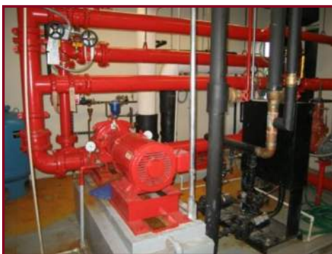
WET PIPE SPRINKLER SYSTEM
