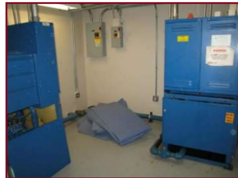
ELEVATOR PUMP CONTROL ROOM
