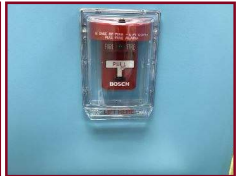
TYPICAL PULL STATION
