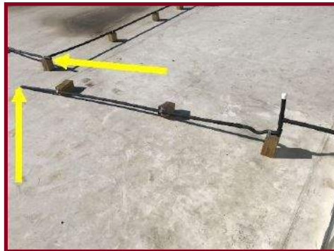
DAMAGED/SEPARATED CONDENSATE DRAIN
