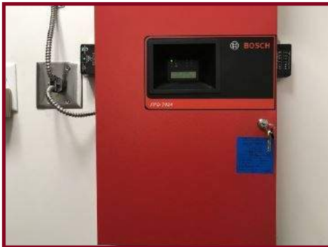
ALARM CONTROL BOX
