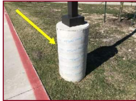
AREA POLE LITE NEEDS SONO-TUBE REMOVED
