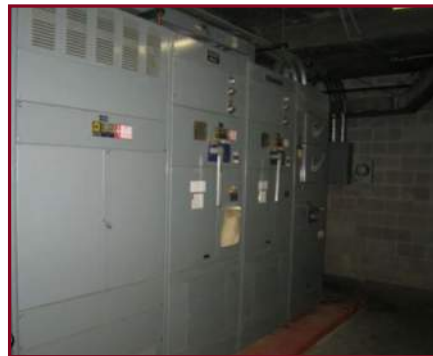
MAIN DISTRIBUTION PANEL
