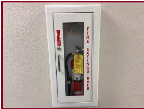
TYPICAL FIRE EXTINGUISHER
