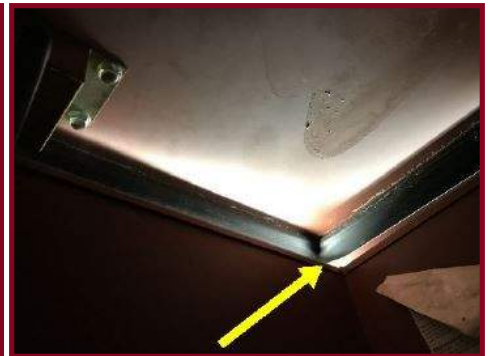
ROOF HATCH DOES NOT SEAL
