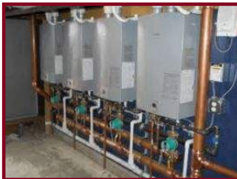
WATER HEATING EQUIPMENT
